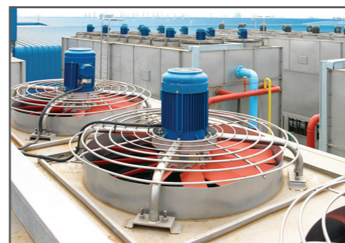
Fans and water pumps
